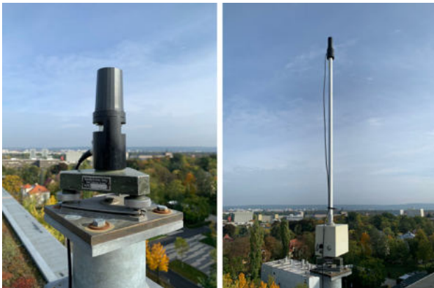
Figure 9: Quadrifilar helix antennas in low and high position.
